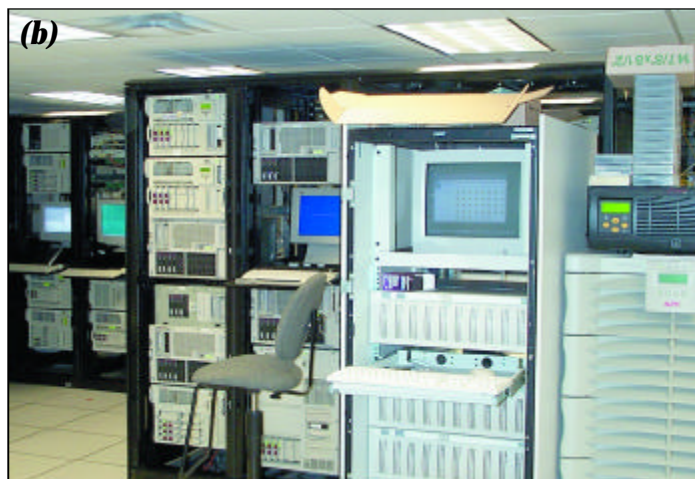
Figure 9. Suncoast Schools FCU's main computer room and the reason for the extensive grounding and surge protection described in this publication. Continuous power to the host computer (a) and various servers and other equipment (b) is assured by means of the stand alone 16-kVA UPS seen at the lower right. Smaller UPS devices are located at individual workstations.
