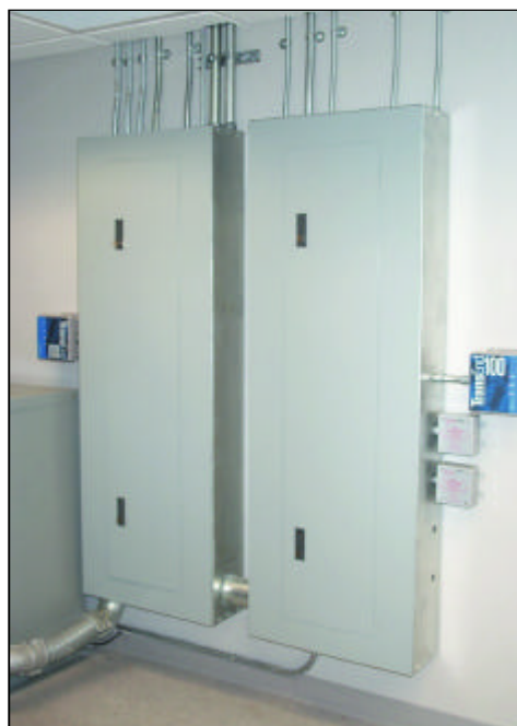
Figure 8. Two 120/208-V branch circuit panels supply the data center's computer room and other locations in the building, respectively. Each panel is protected by TVSSs rated at 100 A (blue enclosures). Fire alarm and fire call circuits are additionally protected by TVSS devices rated at 20 A. There are as many as seven layers of surge protection in critical portions of the data center's electrical system.
