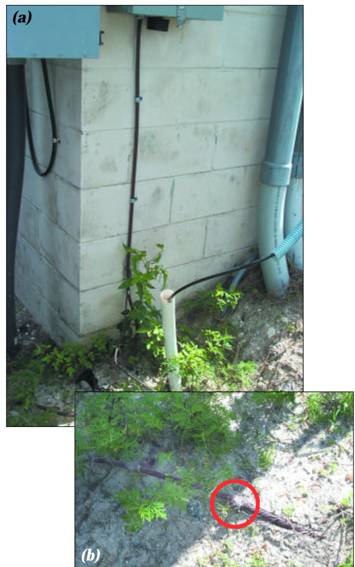
Figure 4a. The main grounding electrode conductor extends from the electrode array to the meter box (vertical cable) and to the service entrance panel seen at upper left. The 4/0 grounding cable leading to the right connects to the air-conditioning equipment subpanel. Exothermic welds ( Figure 4b ) connect the grounding electrode conductor to other outdoor equipment.
