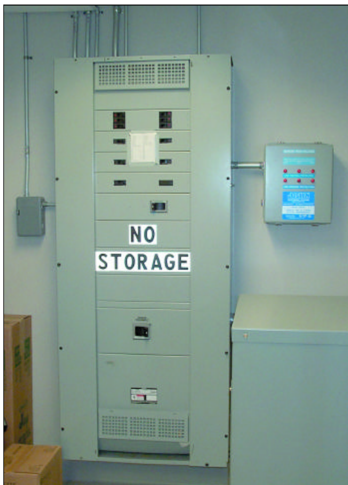
Figure 7. The 480-V distribution panel shown here feeds a 480Δ – 208Y/120-V transformer (lower right), the 277-V lighting circuit and the two air conditioning units. Connected to the 480-V bus at the right side of the panel is a 200-kA-rated TVSS that provides both line-ground and neutral-ground protection.
